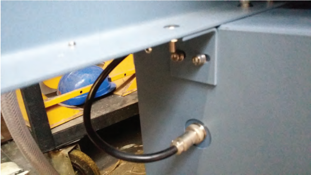
Picture No.9 - Plug in electrical connection
